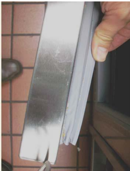
Gasket in good condition
