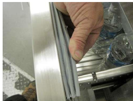
Check to see if the door gasket is in good condition
